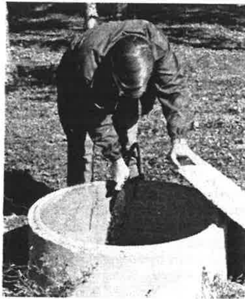
Fig. 3. Strong chlorine solution is recirculated back to the well.
